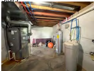
Mechanical in basement
